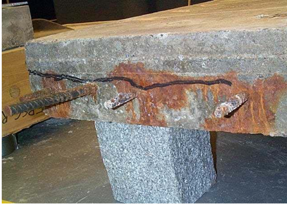
Figure 12.21 Crack in the corner of the slab resulting from the expansion of the rebar during due to corrosion.
