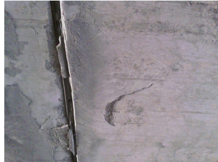
Visual of Delamination
