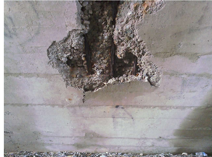
Visual of Delamination
