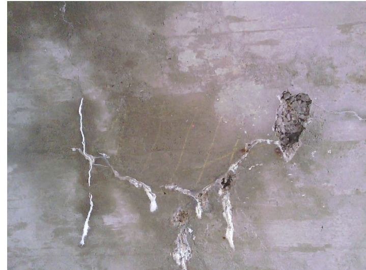
Visual of Delamination
