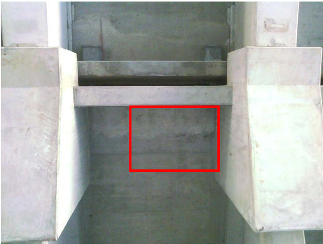
Visual of Delamination
