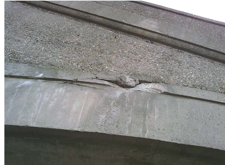
Visual of Delamination
