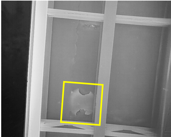
Figure 53 - Delamination without Visible Separation
