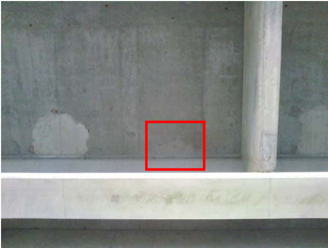
Visual of Delamination
