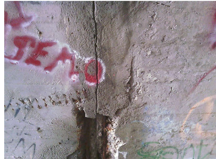
Visual of Delamination
