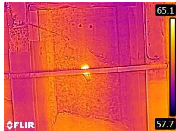
Figure 33 - Pigeon affecting Thermal Span
