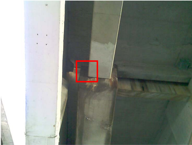
Visual of Delamination
