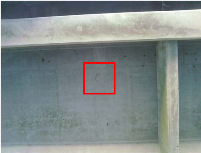
Visual of Delamination
