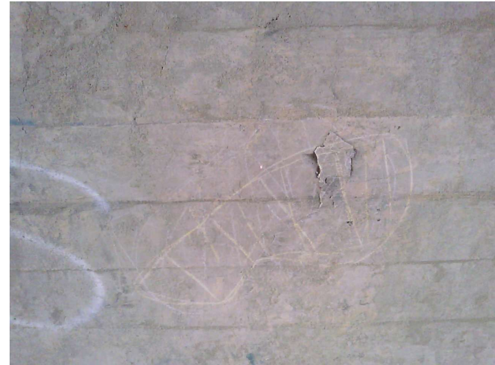
Visual of Delamination
