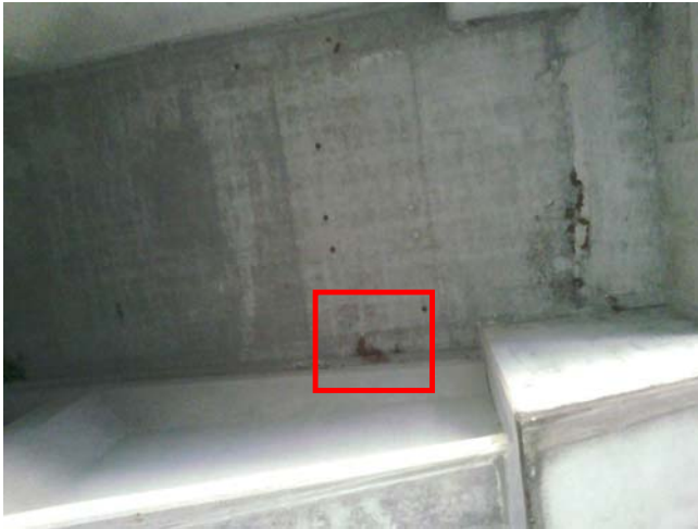
Visual of Delamination
