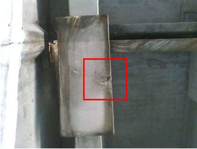
Visual of Delamination
