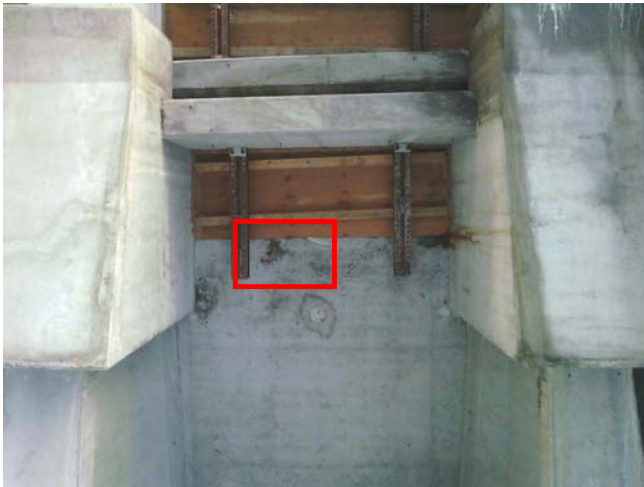
Visual of Delamination
