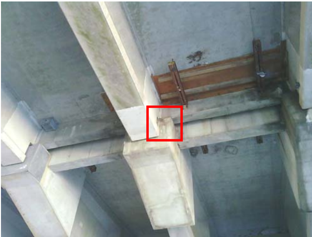
Visual of Delamination
