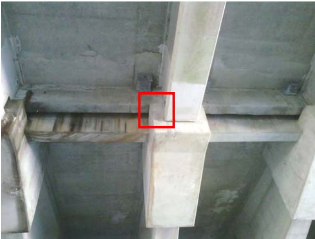
Visual of Delamination
