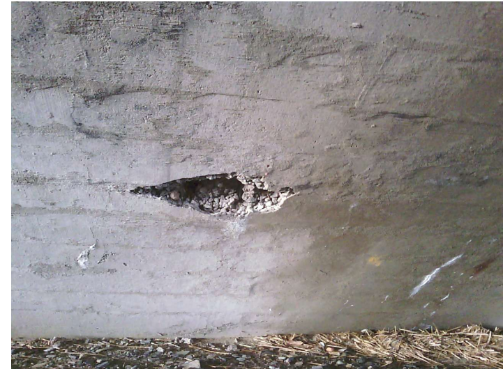
Visual of Delamination
