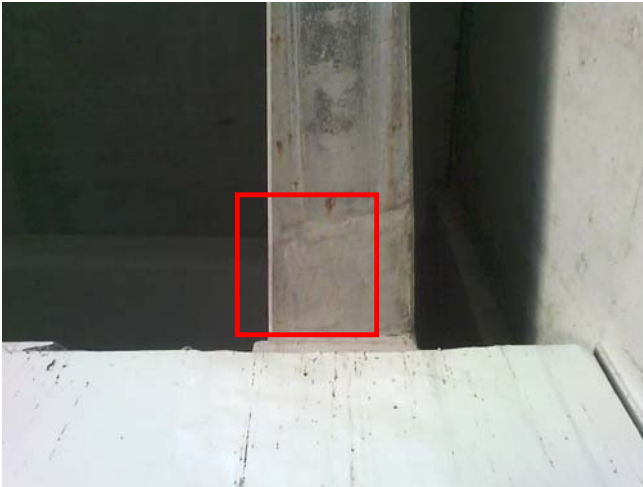
Visual of Delamination
