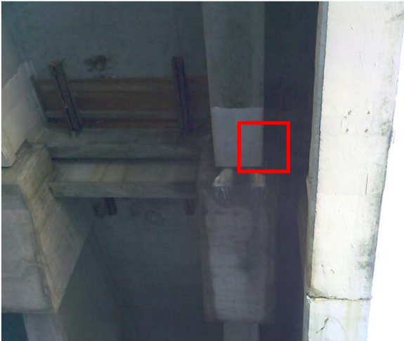
Visual of Delamination
