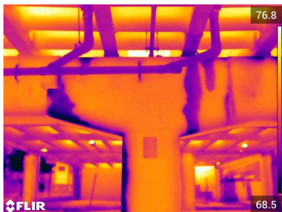
Figure 34 - Water Leakage affecting Thermal Span
