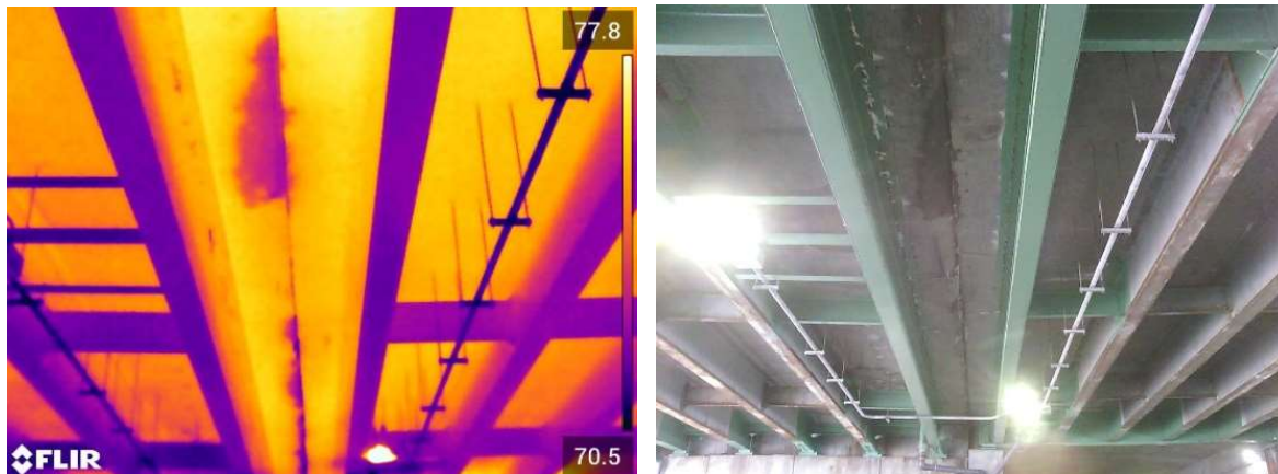
Figure 45 – Temperature Differential caused by Leakage along Joint
