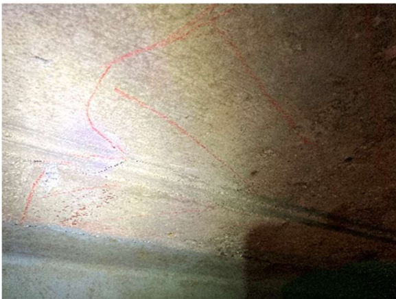
Figure 68 - Delamination from Thermal Survey
