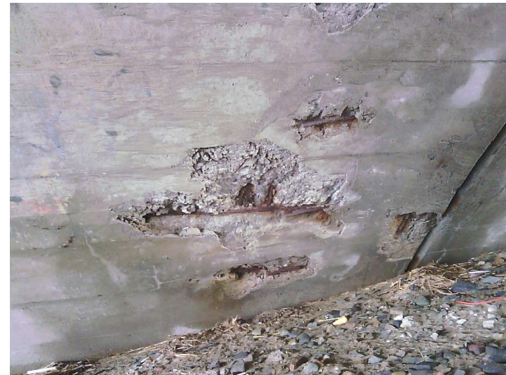
Visual of Delamination
