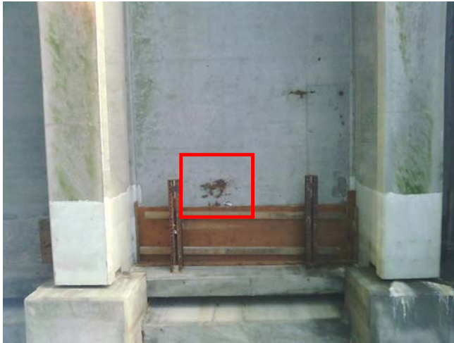
Visual of Delamination
