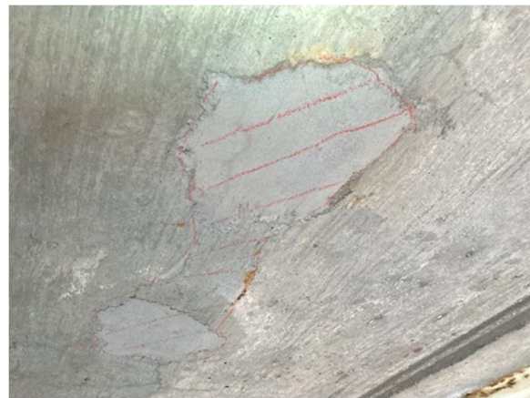
Figure 67 - Minor Delamination from Thermal Survey
