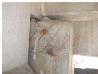
Figure 74 - Delamination at Top of Vertical Face of Cantilever
