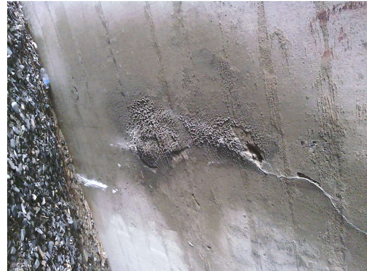
Visual of Delamination
