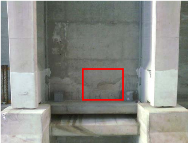
Visual of Delamination
