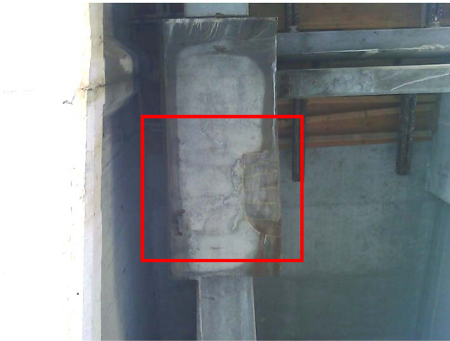
Visual of Delamination
