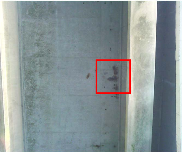
Visual of Delamination
