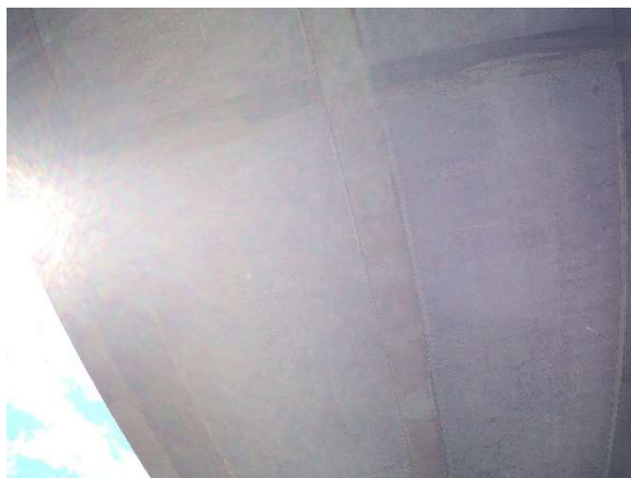
Figure 48 - Sun Glare obscuring Deck
