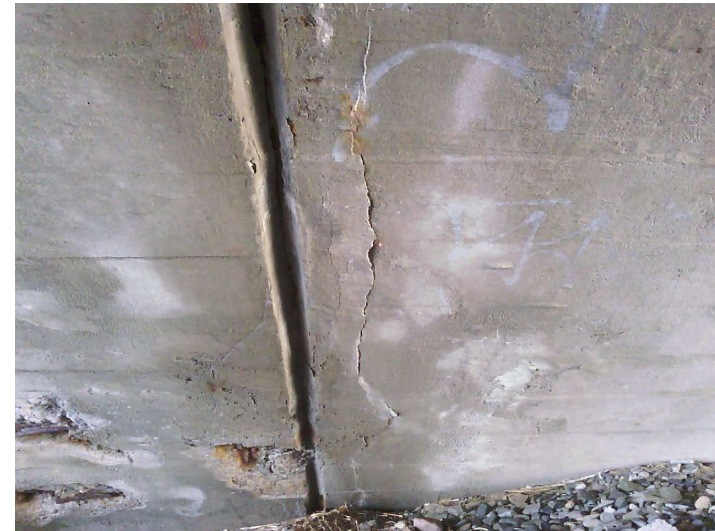
Visual of Delamination
