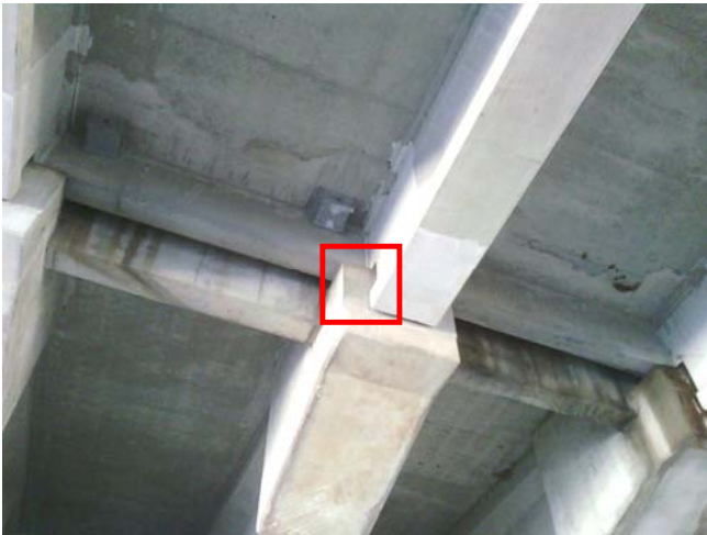
Visual of Delamination
